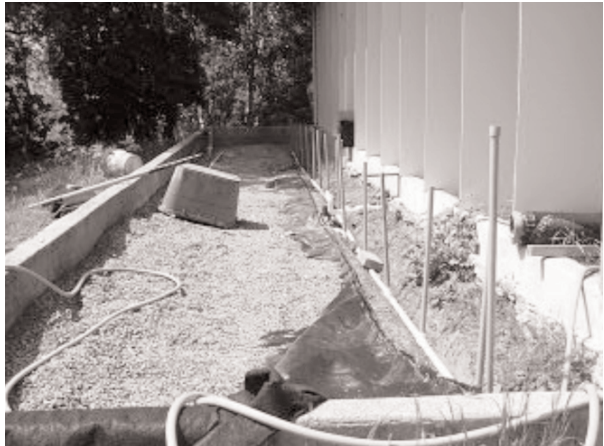
Picture showing the water main line with the services coming up at each flight. This area gets covered with gravel to within 2' of the foundations.
